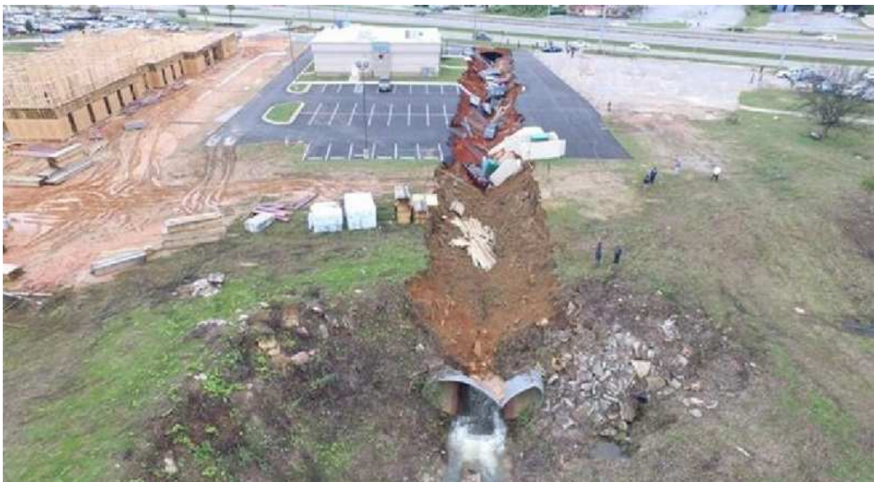
This 400' long CSP failure is still fresh in minds of many residents of Mississippi. It happened instantly once the soil structure around the pipe was disturbed. Thankfully no one was hurt.
