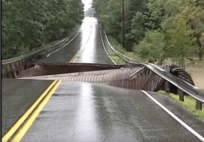
This lightweight CSP was washed away from a rainstorm, blocking essential access for road users
