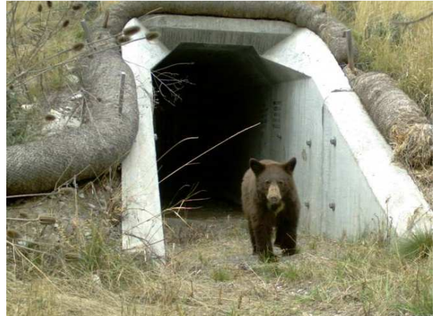
In addition to conveying storm water, culverts are also designed as wildlife crossing.
